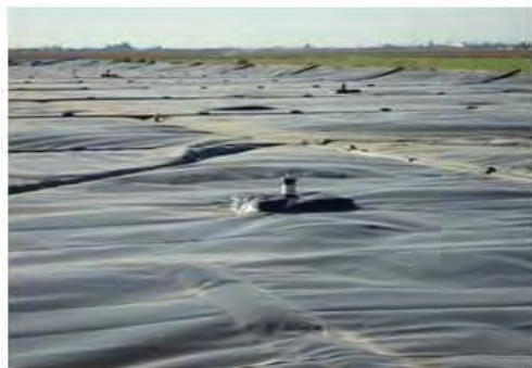
Covered Lagoon Digester
