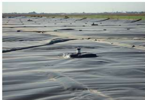
Covered Lagoon Digester
