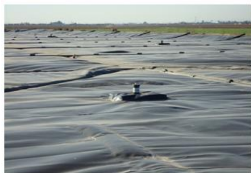
Covered Lagoon Digester
