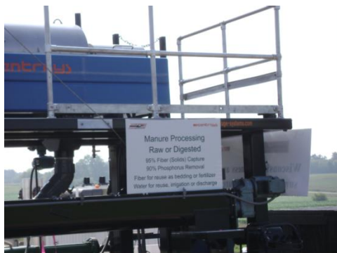
Pumping and Processing Equipment
