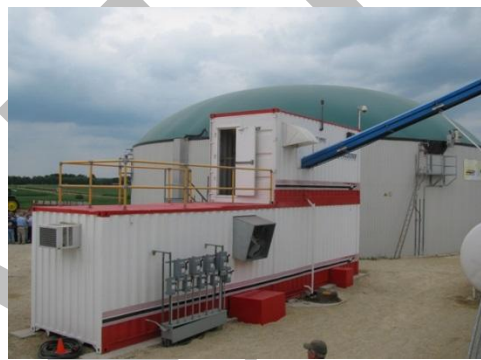
Gasifiers and Digester Tanks
