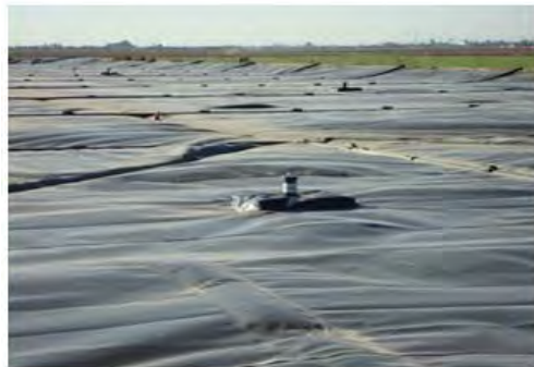
Covered Lagoon Digester
